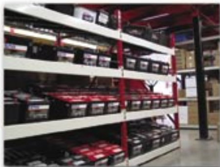
Battery Storage Units
